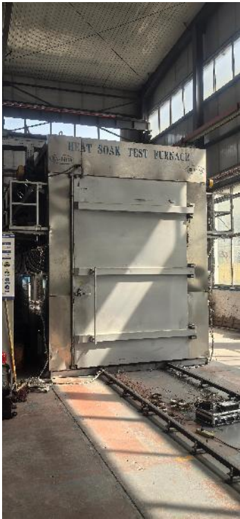
Fig.2 Heat Soak oven of Shandong Lanjing Glass Technology Co., Ltd.
